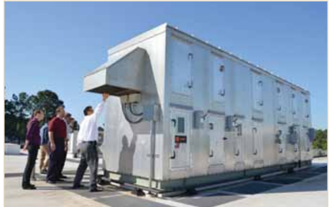
The dedicated outdoor air system.
