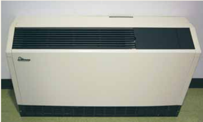
One of two ClimateMaster Tranquility® Console (TRC) Series units installed in ASHRAE headquarters.
